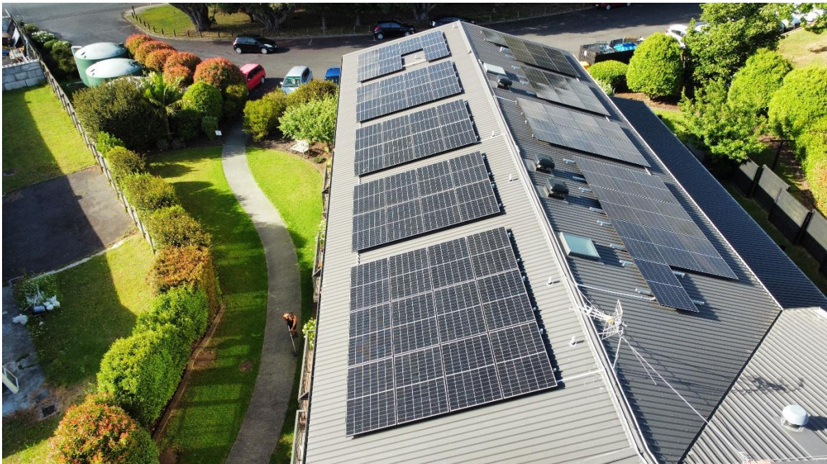
Part of the solar array installed on the Merrivale Retirement Village in Whangarei
