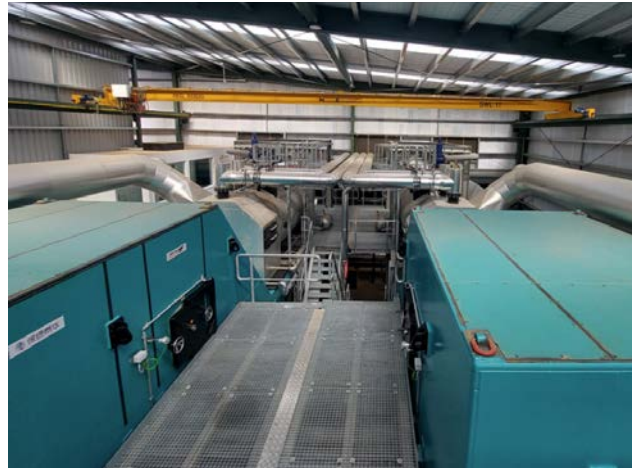
Figure 14: Top View of Boiler Furnaces
