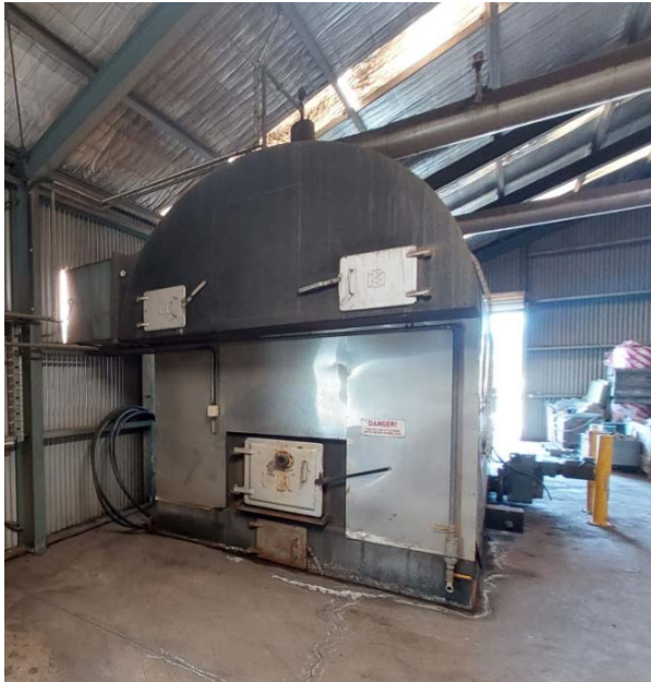
Figure 3: Example of Old Fire-tube Coal Boiler
